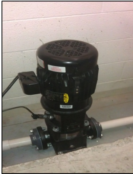
Figure 3.3 Network supply recirculating pump
