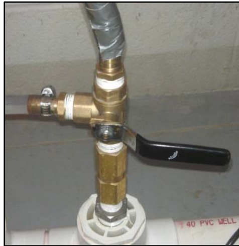
Figure 3.5 Injection line flow control valve
